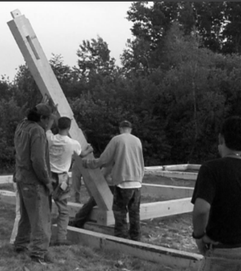
The beams of Rice Hall were fashioned as part of a community timber framing class led by Tim Beal in the early 2000s and the frame was raised in April 2004.
